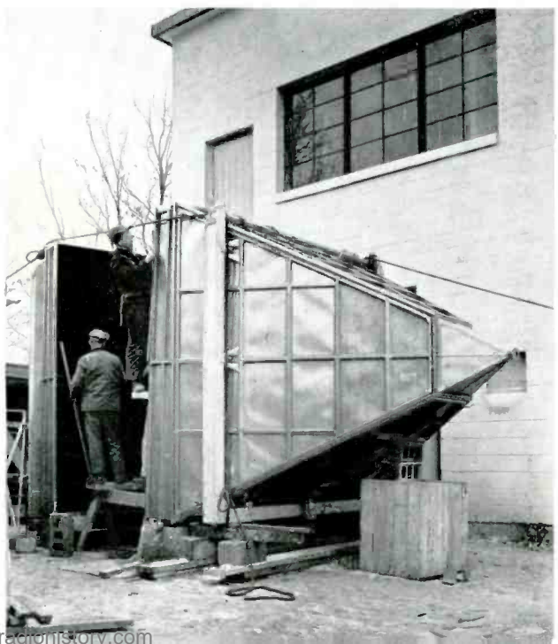
4. Antennas being assembled. By December, these metal lens antennas designed by Bell Telephone Laboratories were ready for hoisting to top of tower.
