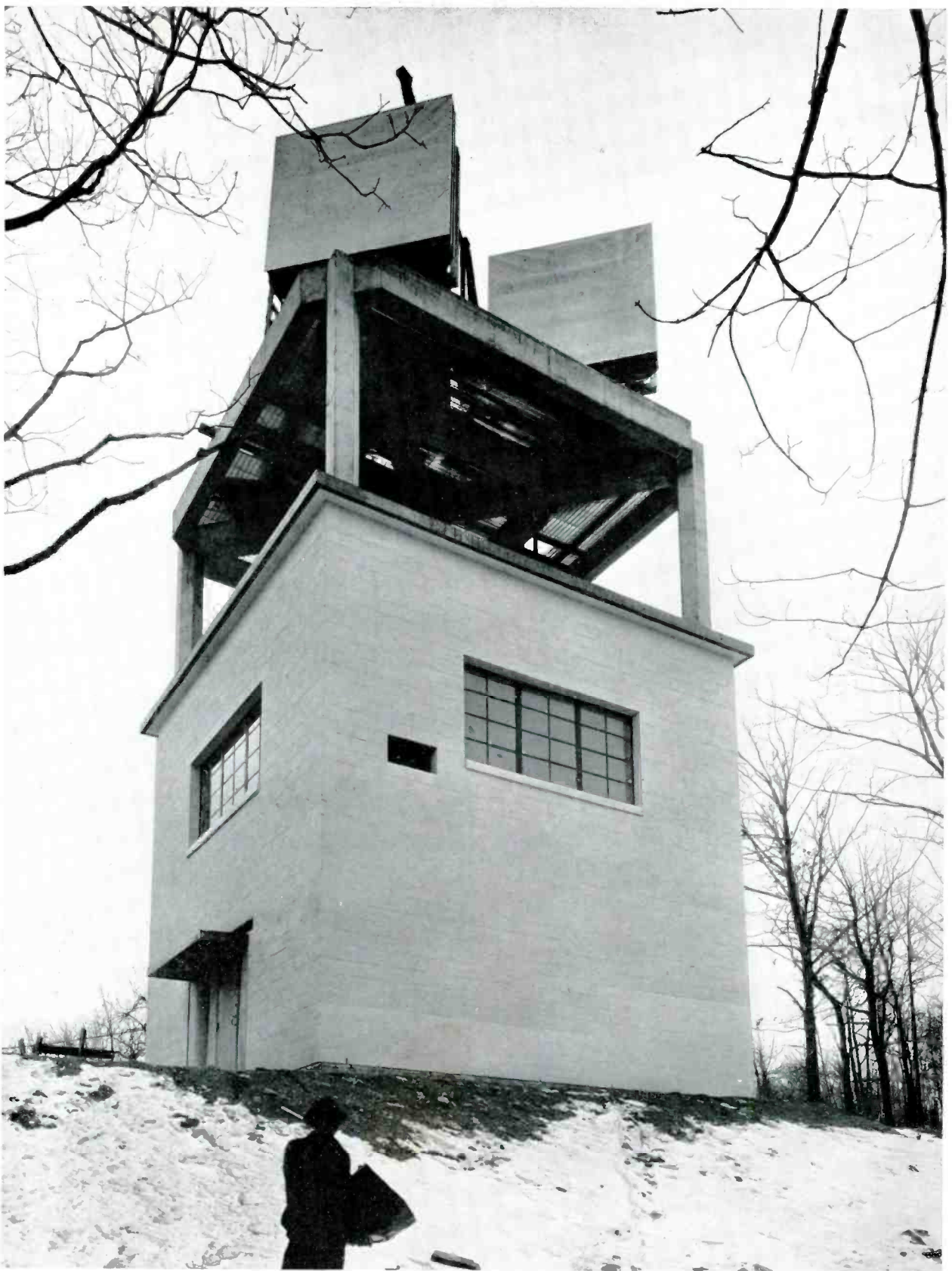
5. Antennas in position. Two of the four metal lens antennas are now in place atop the tower. The next step is the installation of the receiving and trans-
