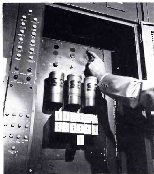
A special relay panel in the "F" unit of the 50 kw transmitter at WHN provides split-second switching from 50 to 1 or 5 kw of power in emergencies.
