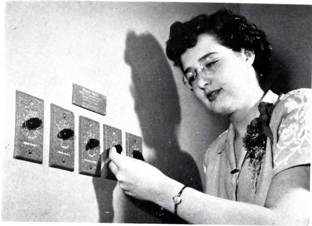
In addition to the main volume controls located on the control unit, additional controls are provided in a corridor near the dining rooms and cocktail lounges to adjust sound levels locally.
