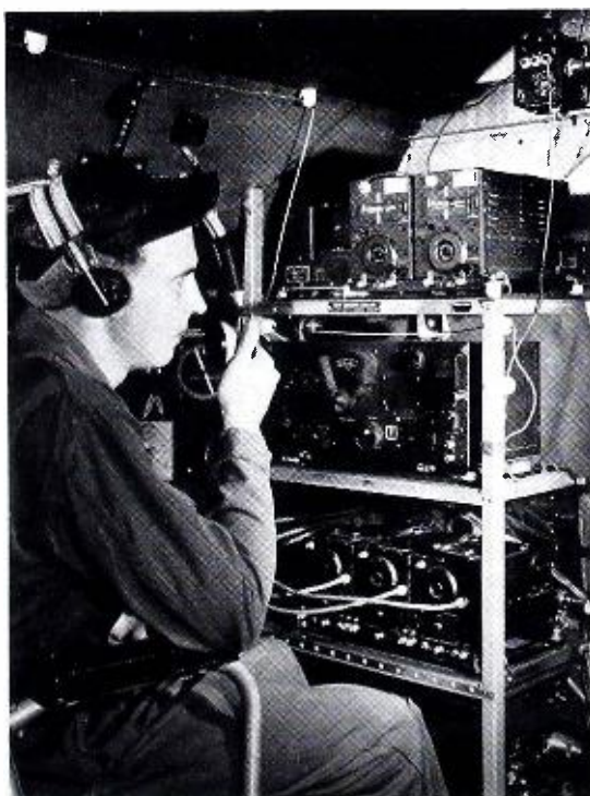
The famous SCR-274 Western Electric made Command set here being operated in a B-26 bomber.
