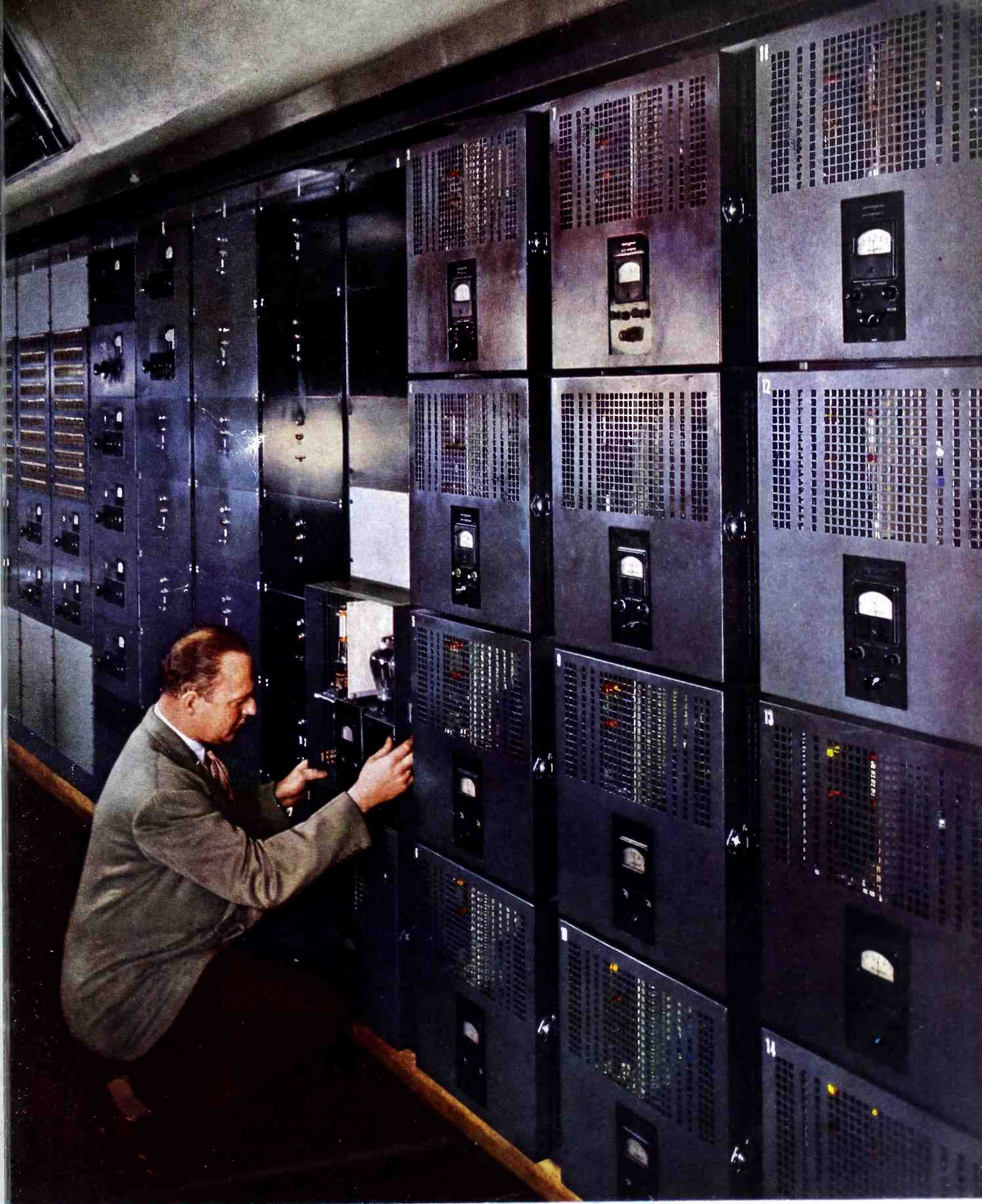
In the New York radio center of OWI, these Western Electric program amplifiers, power amplifiers and driving amplifiers — 46 in all — serve the 14 high fidelity transcription recording lathes.
