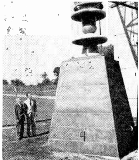
E. A. Merryman and J. W. Anderson, Electronics Field Engineers, inspect base and insulator mountings of the 800 foot tower.
