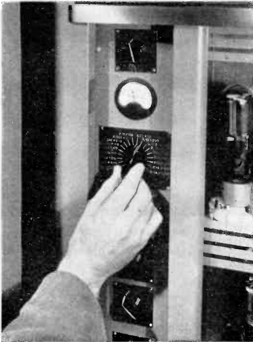
Figure 5. An important maintenance "tool" is familiarity with test point voltages established for normal operation, as read on built-in panel multi-meter.
