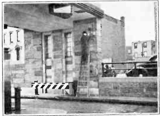
G-E photoelectric installation at entrance of vehicular tunnel as height indicator. When truck is high enough to interrupt beam, loud horn is sounded, warning traffic officers to halt truck. At Queens-Midtown Tunnel, New York.
