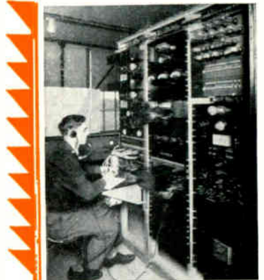
Speech input control panels, Deal Beach Station, for trans-Atlantic Radio Telephony.
