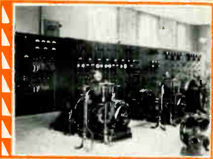
Power Apparatus Room, showing main control switchboard of the Drummondville Station
