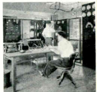
Courtesy General Electric News Bureau General view of W2XAF—experimental relay short wave broadcasting station operated by the General Electric Company.
