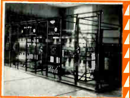
Rectifiers for English and Australian transmitters, Drummondville Beam Station, one of the powerful stations used for commercial communication with countries on the other side of the Atlantic
