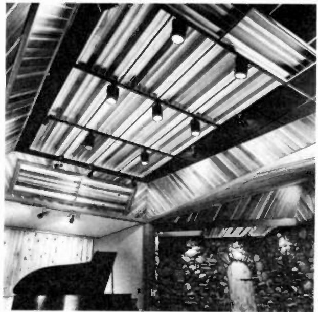
Figure 14. RPG "T-bar" suspended ceiling at BlueJay Recording Studios, Carlisle, MA, integrates diffusion, absorption and lighting.
