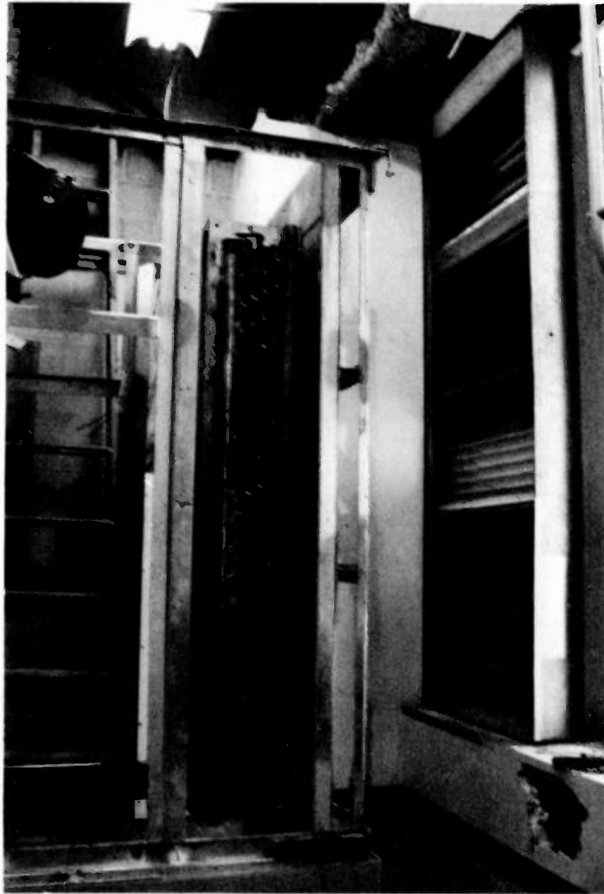
PHOTO - 1 This picture shows a side view of the dry cooler heat exchanger before the blower and covers were installed. The dry cooler was being moved into position for ducting connections to the outdoor air louver. The heat exchanger coil is 2 ft. wide by 6 ft. high.
