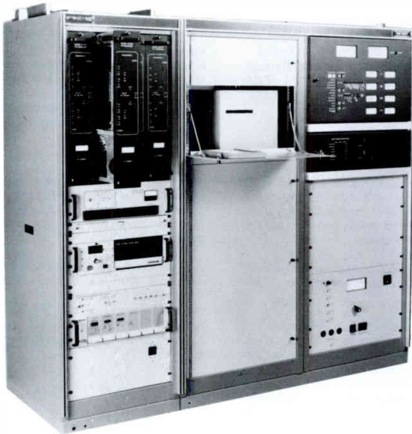
Figure 5. 30kW Single Tetrode UHF Television Transmitter showing solid state driver (left) and PA cabinet center and right
