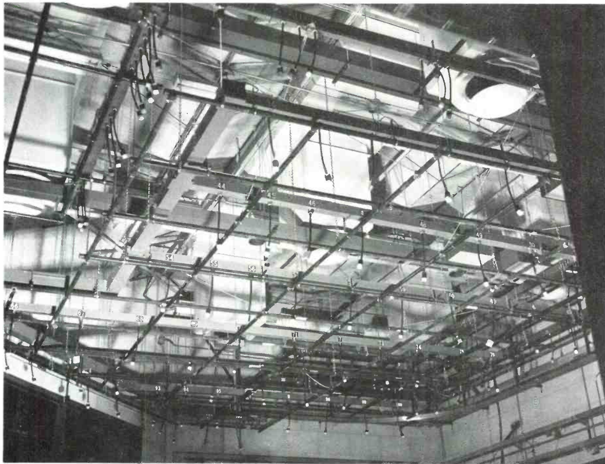
Fig. 3. This fixed grid studio employs two levels to create a higher apparent background, multiple pigtail outlets are positioned for cyc lighting units. (WFAA-Dallas)
