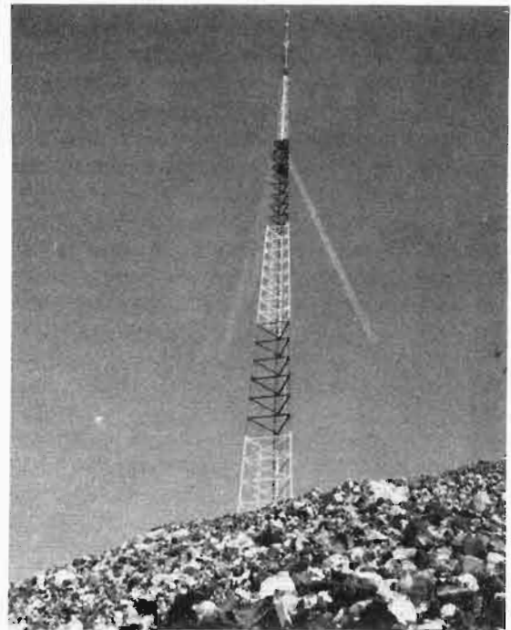
Fig. 4. Spreader array, TV station.
