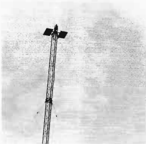
Fig. 3. Panel array, AM broadcast station.
