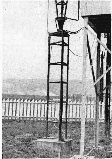
FIG. 2-41. Example of raising base insulator for flood-water conditions.
