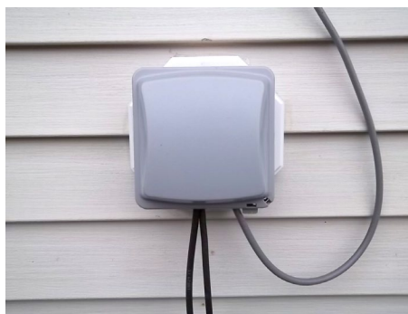
Photo 3. Plastic enclosure, purchased from a big-box store, makes a neat entryway for cables.
