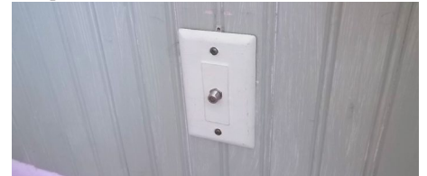
Photo 4. Wall plate with F connector for attachment to FTA radio. Tidy installation keeps me in the XYL's good graces.
