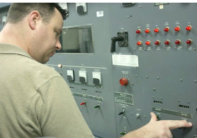
Technician presetting the tuning controls of a GE 250 kW transmitter for the next operating frequency
