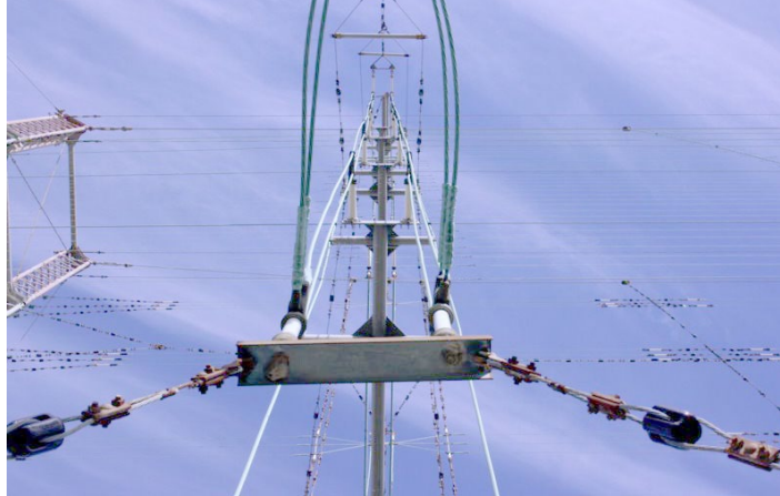
Feed line manifold feeding the dipole elements of a curtain antenna
