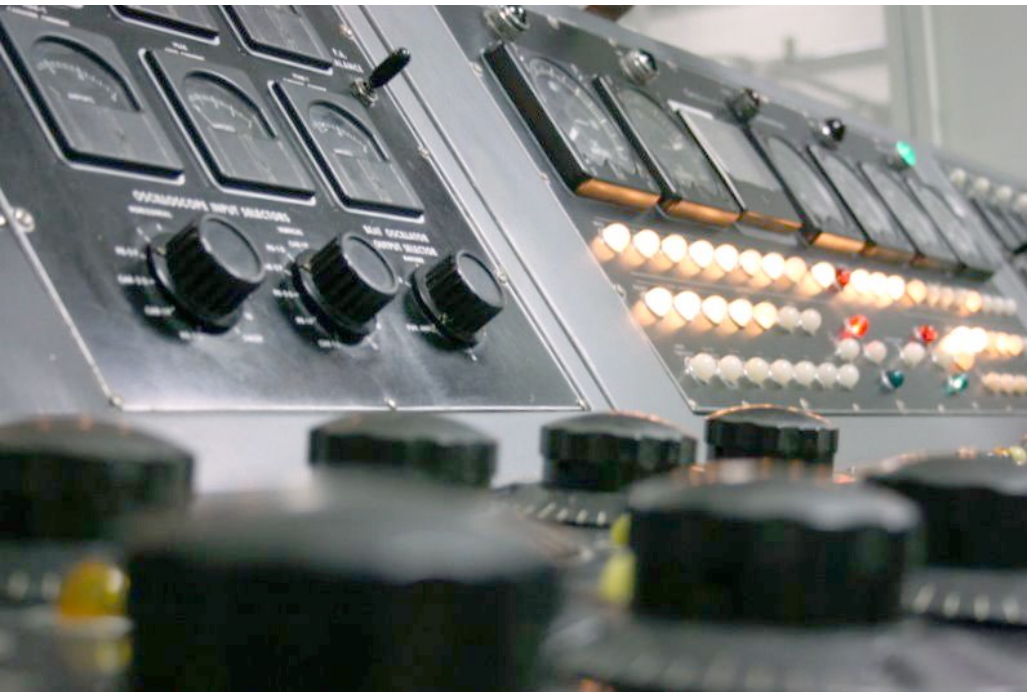
Tuning controls of a Continental Electronics 500 kW transmitter
