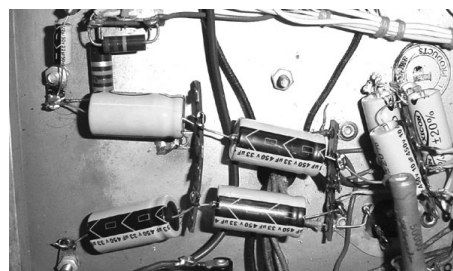
In this shot, all eight of the 680's electrolytics have been replaced. The group of four mounted on terminal strips at center replaces the taped-together pairs shown in the "before" picture.
