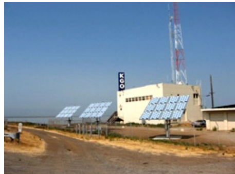
San Francisco's KGO-AM gets help from the sun with its 12 KW solar installation, the first of what the station hopes will be "many new green initiatives." (Courtesy: KGO-AM)
