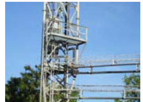
The base of the WBIR-TV tower in Knoxville, Tennessee, shows two horizontal towers used to support feedlines going into the transmitter building.
