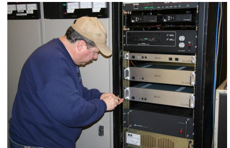
Drew KC2JPP installing 1.2 GHz Voice/Slow Speed Data Module
