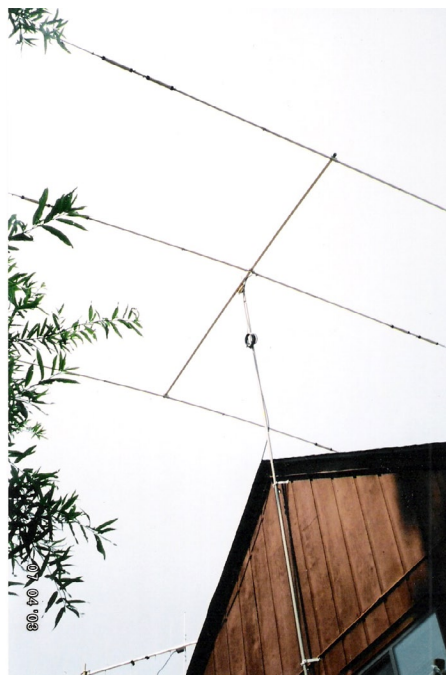
DIY no-tower tower uses three lengths of 10-foot TV antenna mast attached to a gable end exterior wall. A ground rod and a cement block at the base complete the installation. (Courtesy: Author)
