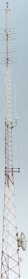
WFOS-FM tower hosts their main broadcast antenna, point-to-point microwave dish for remote broadcasts and local amateur radio repeater antennas for 2 meters and 70 cm.
