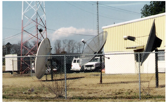
Dish farm at WFOS-FM with the base of their free standing 172' broadcast tower. Just out of the picture is the 30 kW propane fired generator shed.
