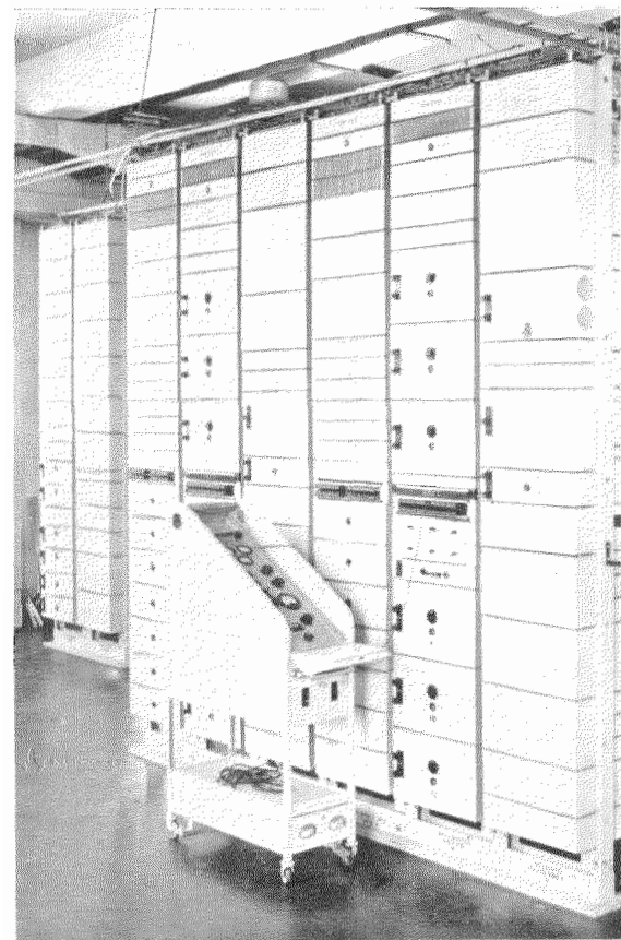
Fig. 10—Part of the Bloemfontein terminal equipment.
