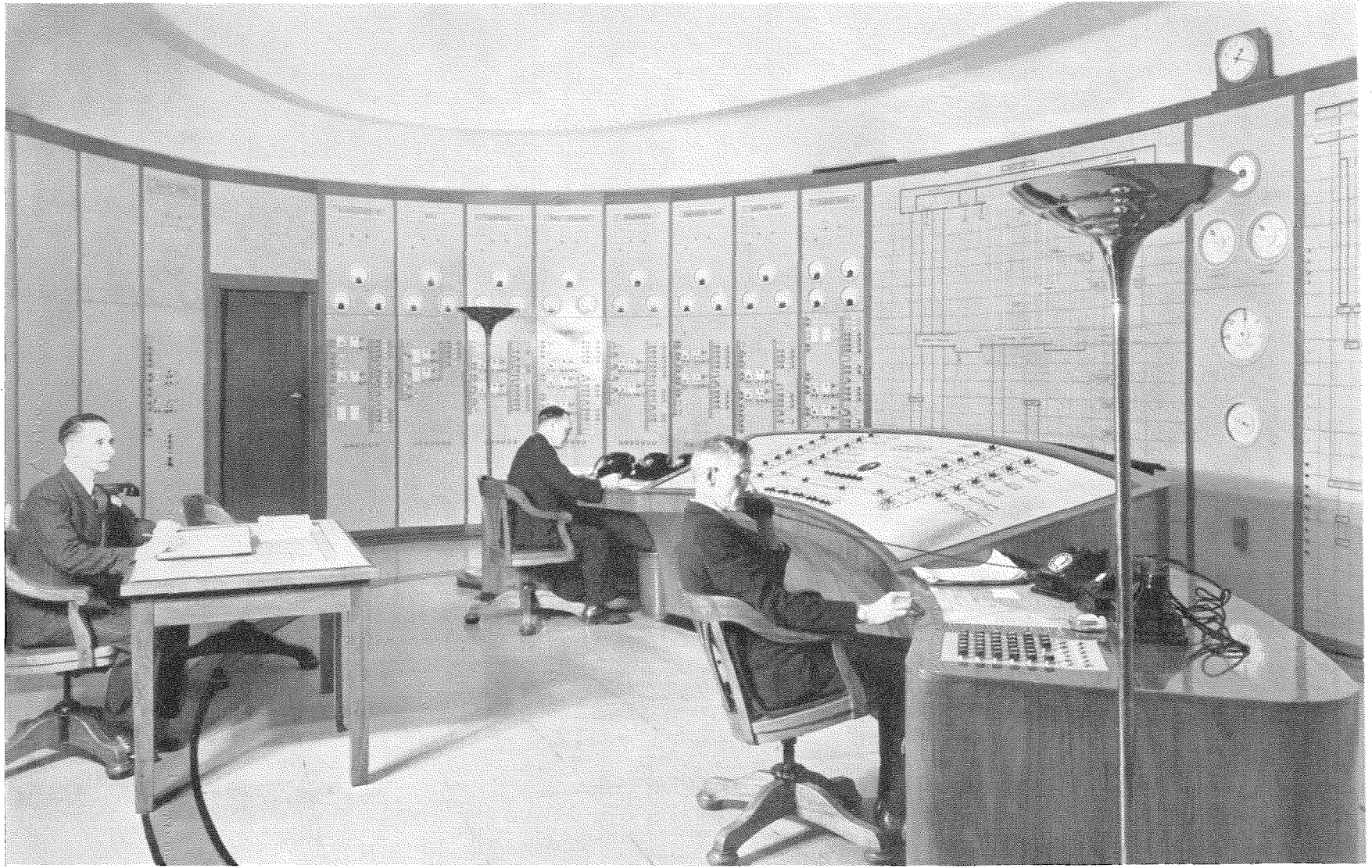
General view of the central control room of the Manchester Corporation Electricity Department. In the background are the panels for the remote control, indication, and metering of nine 33-kilovolt main substations. To the right of these is the 33-kilovolt system diagram separated from the 6.6-kilovolt diagram, shown in part on the extreme right, by a central loading and frequency panel.
