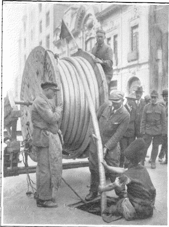
Feeding 2424 Pair Cable into manhole, Bucharest, Rumania. This cable, containing the largest number of pairs ever manufactured commercially for a customer in any country in the world (1932), was supplied by Standard Telephones and Cables, Ltd., London.
