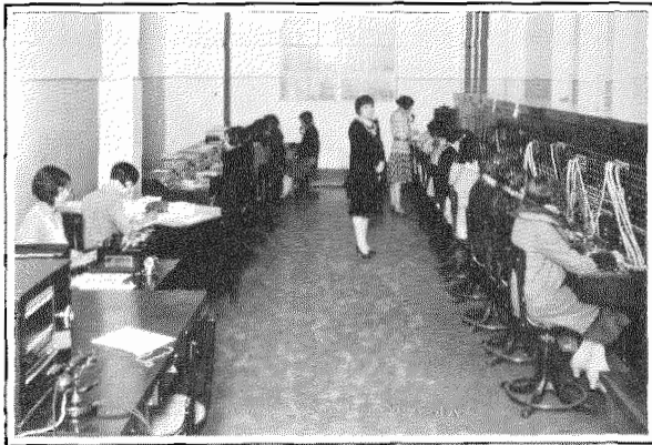
Operating Room in Principal Central Office Showing Chief Operator's Desk, Complaint Desk, Time-of-Day Position and Toll Switchboard.
