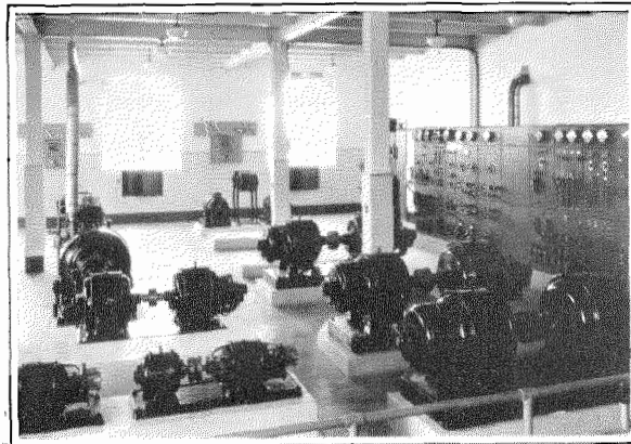
Power Room, Principal Central Office.
