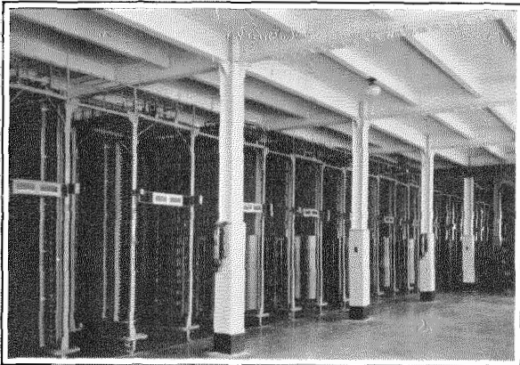
Switchracks in Principal Central Office.
