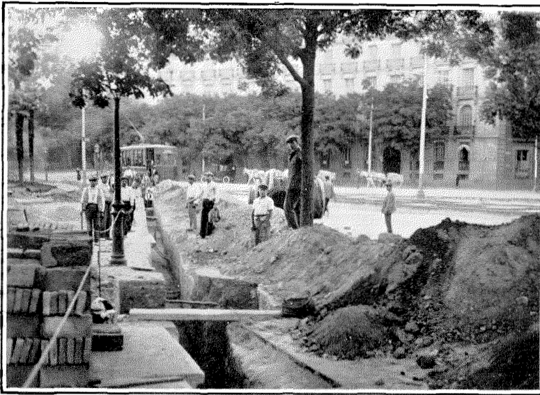
Figure 5—Running a Trench of the Underground Telephone Cable System across the Plaza Colon, Madrid. The variety of pipes and bare cables of other subterranean systems crossing at various levels may be noted.
