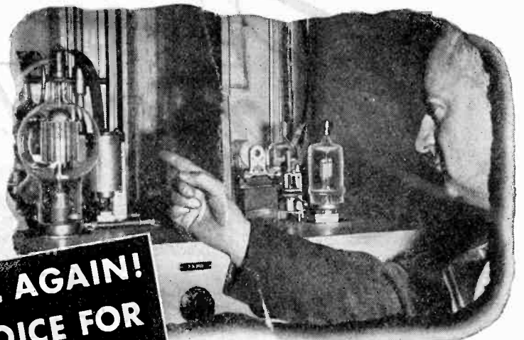
Mr. Brolly calls attention to the Eimac 1000-T's in the final stage of the Audio FM Transmitter which operates at 65.75 megacycles. It is a very stable amplifier of good efficiency.
