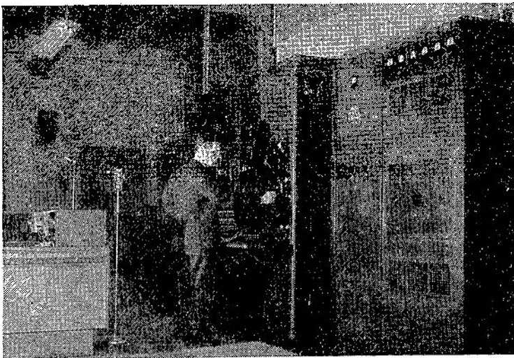
The frequency-modulated-wave transmitting station, W2XOR, which will be open for inspection during the Convention. The control desk may be seen at the left.
