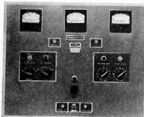
Front view of the phase monitor, showing antenna current ratio meters (upper-left and center) and combined null-indicating galvanometer and test meter. Rotary source selector and testing switches are located on the center-left and the direct-reading, 360-degree phase indicating dial appears through the small center window
