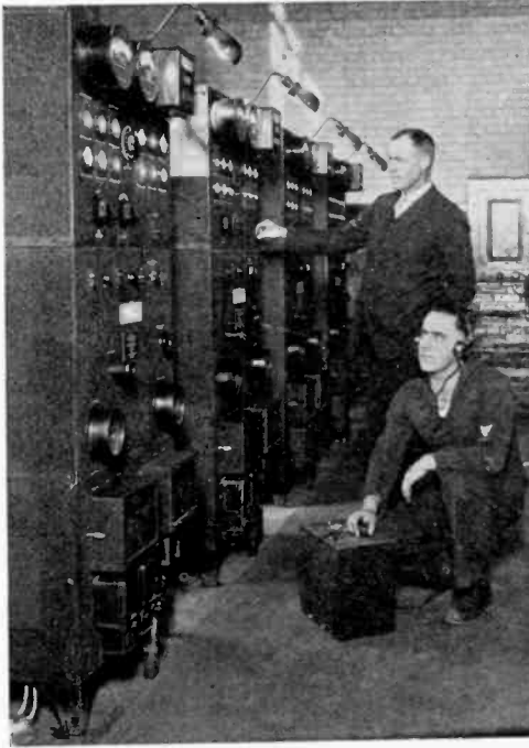
Bank of Four High-Power High-Frequency Transmitters at Arlington Radio Station (Trip No. 3)
