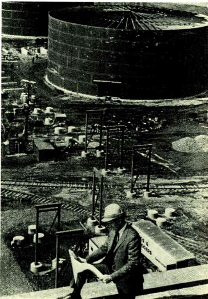
FIGURE 5. Construction superintendent on Ridgeland Station conversion project checking work progress from roof of this power plant, which is being converted from coal to the burning of low-sulfur oil. In the background are two of the four 4-million-gallon (14-million-liter) new fuel-oil storage tanks.
