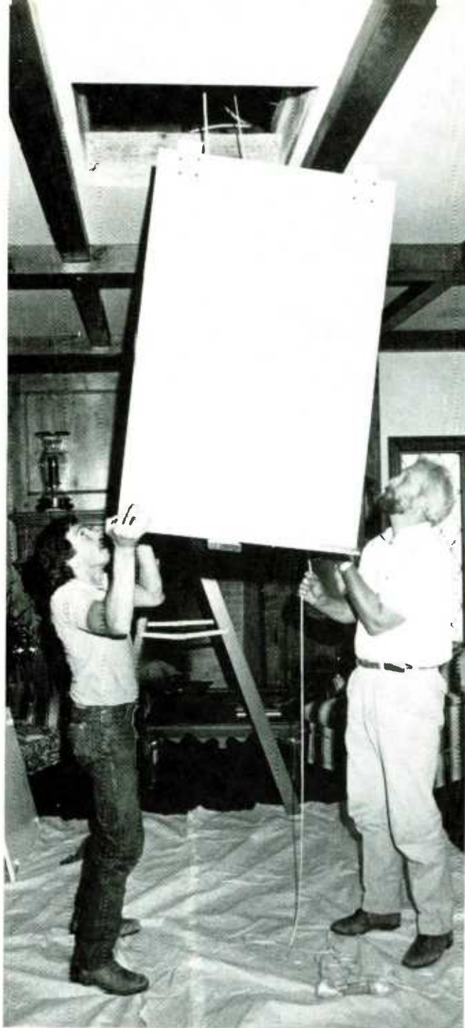
Walin and his assistant fit the television projector platform into the ceiling at the Venuto house. It will be raised and lowered by a pulley system.
