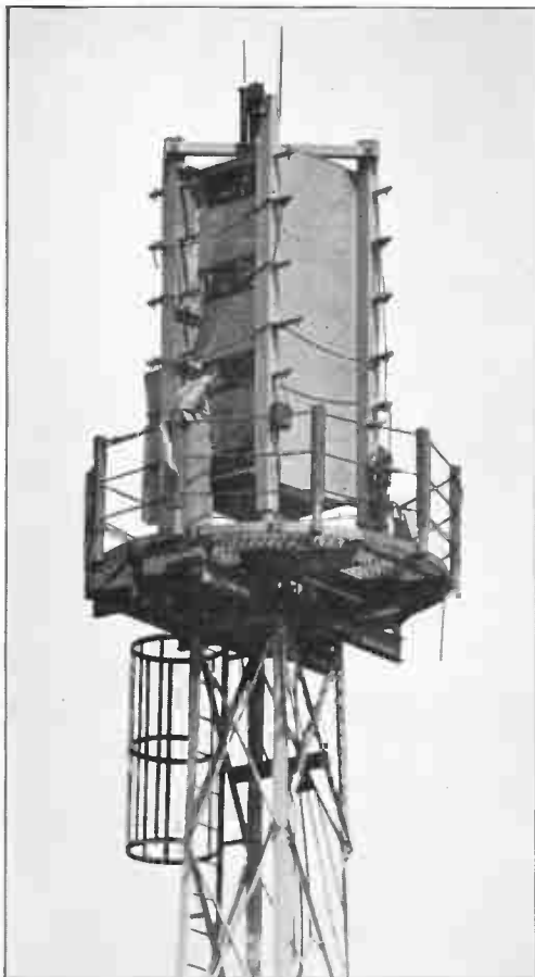
G. E. TELEVISION RELAY ANTENNA AT SCHENECTADY, BEFORE IT WAS COVERED BY WOOD HOUSING AS PROTECTION AGAINST WEATHER
