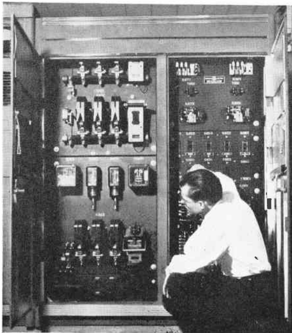
FIG. 7. CONTROL EQUIPMENT AND PROTECTIVE DEVICES FOR THE 50-KW. STATION
