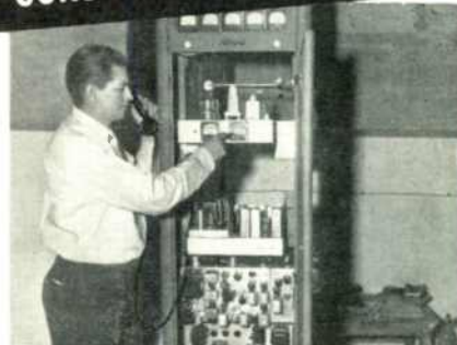
Typical Motorola transmitting and receiving unit as installed for Miami Police Department.
