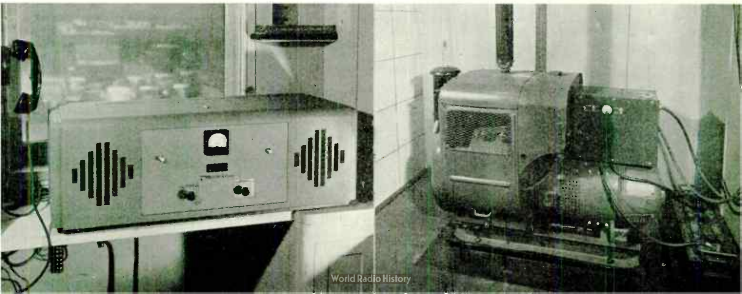
FIG. 3, LEFT: FM TRANSMITTER-RECEIVER IN THE OPERATING ROOM. FIG. 4, RIGHT: THE 5-KW. AC POWER PLANT FOR 115 VOLTS
