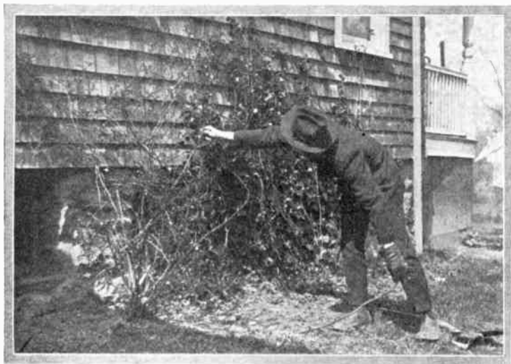
The ground wire runs from the instruments to the plot, and is soldered to the network in the ground.
