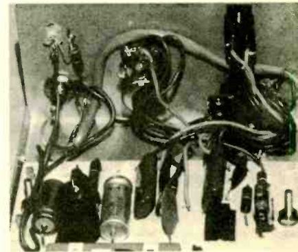
This photo shows the soldering connections at the rear of OSCAR's front cabinet panel.
