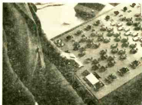
Engineer stands before central control board of Odeillo's mirror-spangled solar furnace.
