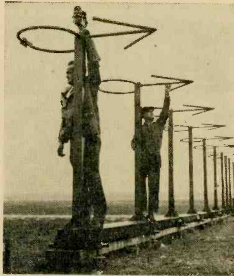
Destined for installation at end of airport runways in some 29 cities across the country, IIT Federal's V-ring antenna array will simplify instrument landings.
