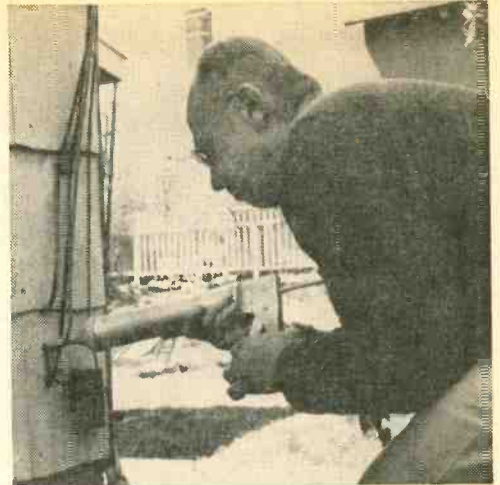
The telephone company has already found the easiest 3 way in through the walls of your house, so drill your transmission line hole, using an electrician's bit, next to the phone line.
