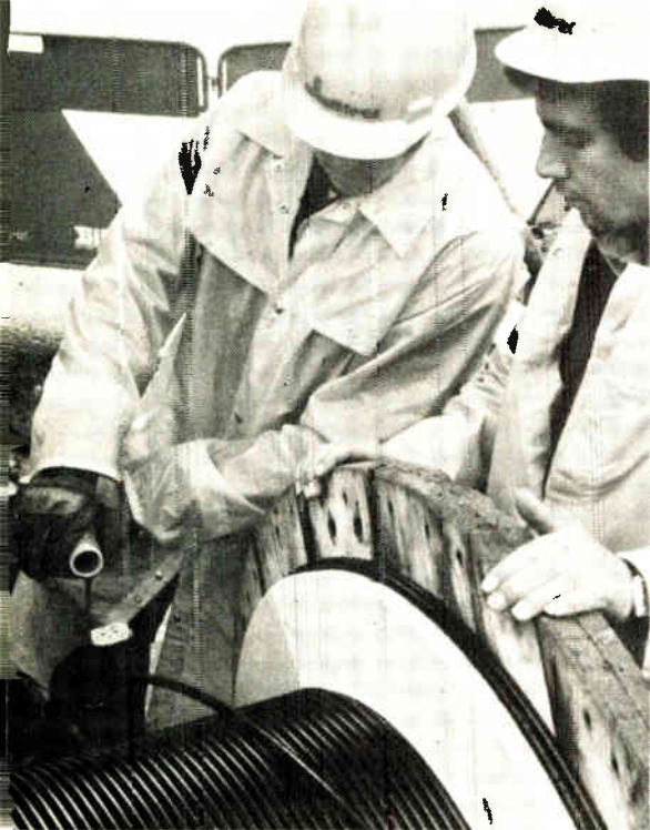
Forging a link. Italian workers unroll fiber-optic cable. Phone network has cut back on spending, so manufacturers look to exports.
