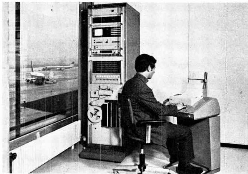
Monitoring noise. At Stuttgart's civil airport, this automatic system samples aircraft noise, prints out details every time pre-set levels are exceeded. Teletype is used to alert authorities to high noise events.
