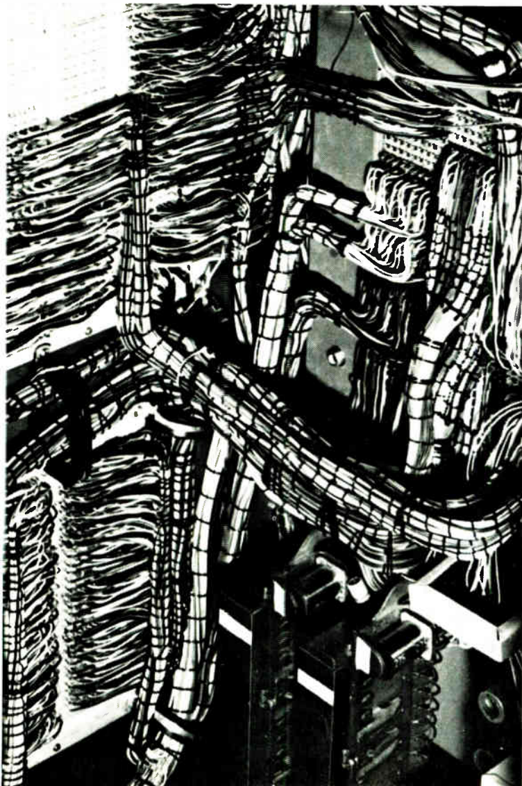
High-density interface wiring with A-MP* taper pin blocks.
