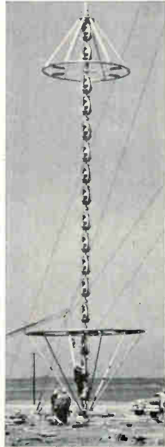
Special antenna insulator assembly with grading rings.
