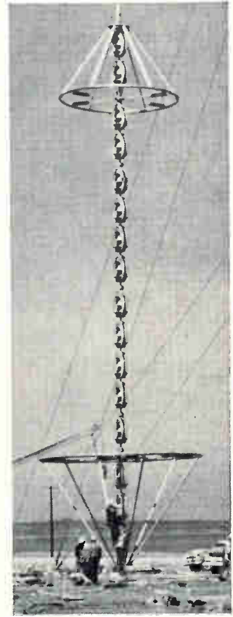
Special antenna insulator assembly with corona rings.
