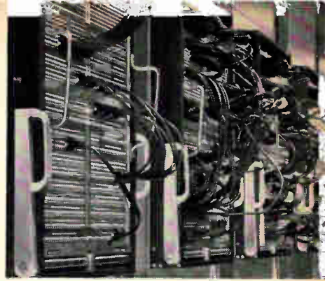
Rocket test data is programmed with AMP's Patchcord Programming System.
