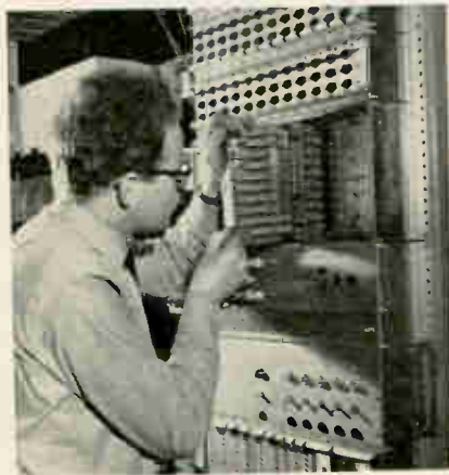
Terminal rack. This unit is part of a pcm system being tested by British Post Office, which administers country's telephone system. Rack was built by Standard Telephones and Cables, Ltd., an ITT affiliate.
