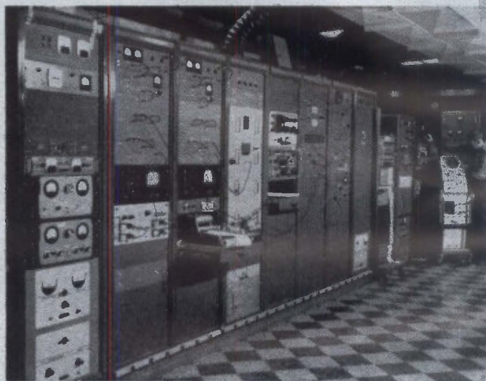
RECEIVER room, containing i-f section and some data processing equipment, is connected by 1,400 feet of coaxial cable to receiver front end located in antenna house
