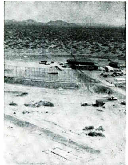
OVERALL VIEW of Nike-Zeus acquisition radar transmitter site at White Sands Missile Range during construction of main fence; auxiliary fence was added later—Fig. 1
