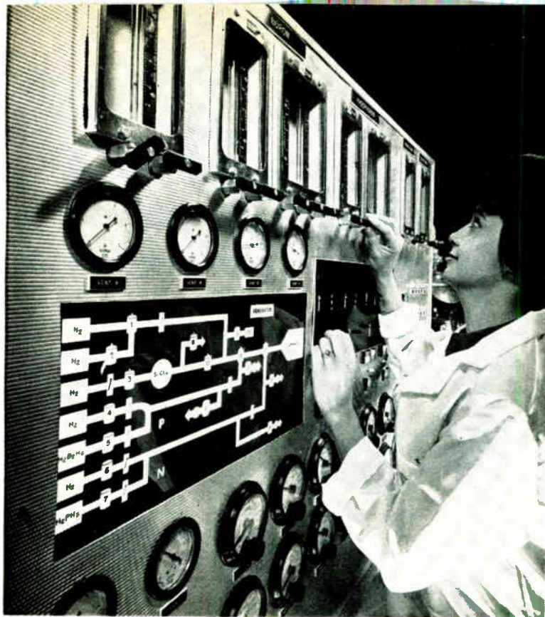
Automatic control panel for epitaxial furnace
