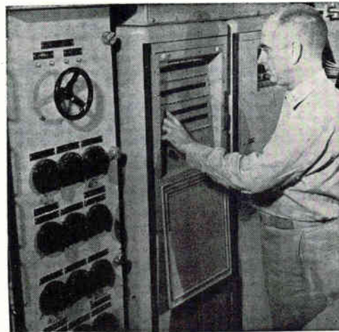
Complete navigation computer, NAVDAC installed on Polaris submarine George Washington. Cabinet design allows easy passage through a submarine hatch
